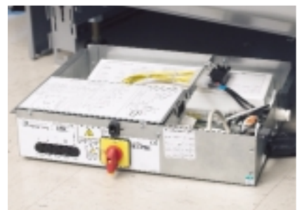
Pull out electrics tray for ease of accessibility
