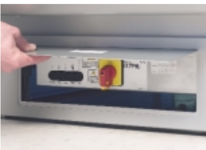
Easy access for electrical isolation
