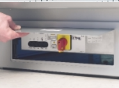
Easy access for electrical isolation
